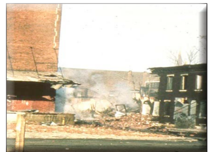
Images 5, 6, 7: During a planned demolition, a vacant, five-story, heavy-timber warehouse flattened the two-story row house across the street. No one was injured because forward-thinking firefighters vacated the occupancy prior to demolition.
